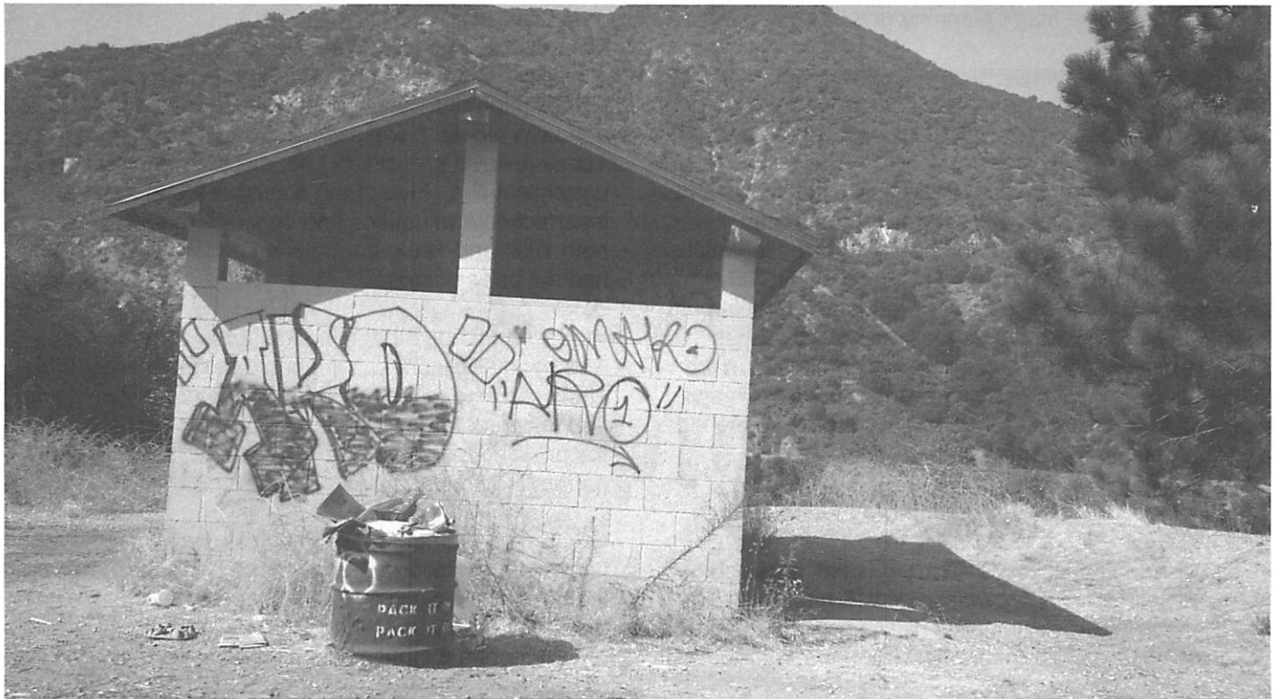
Vandalism and other maintenance needs have outpaced FS resources in certain areas. OIG photo.
