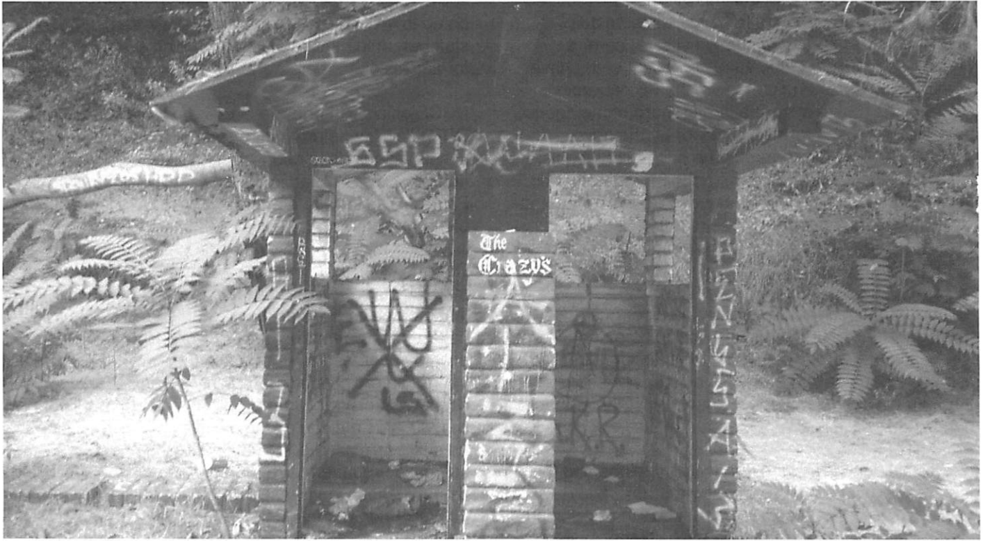
Vandalized restroom at Mt. Baldy Ranger District. OIG photo.
