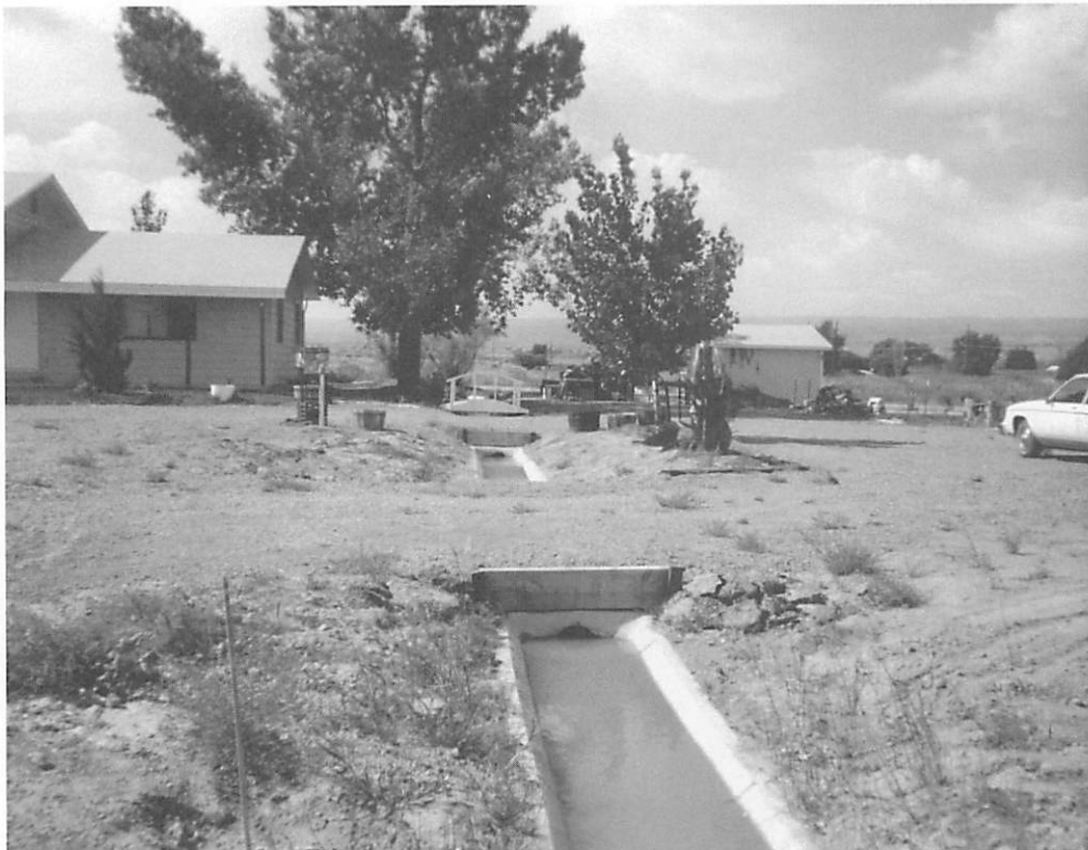
Construction costs for new home driveway culverts were shared inappropriately by USDA. OIG photo.
