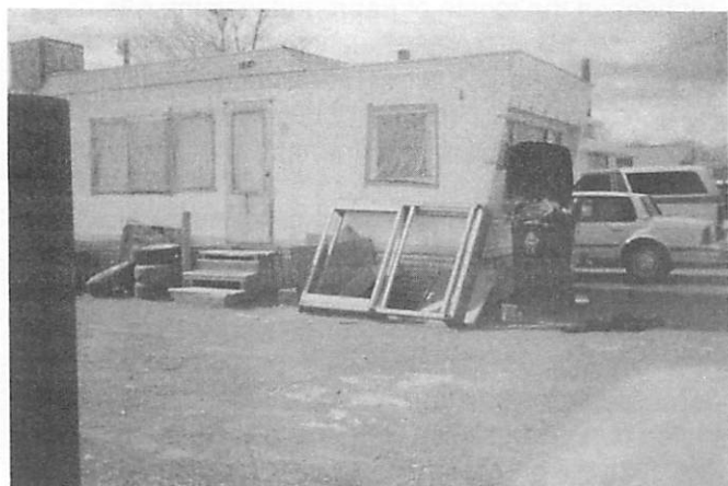
During our "sweep" in Utah, we found that this trailer was being used to provide day care. OIG photo.
