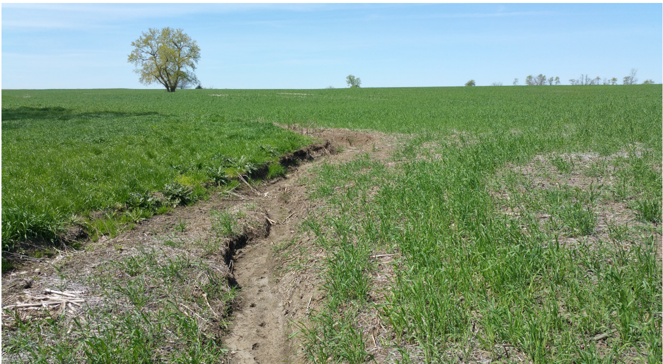
Figure 5: This producer used an approved conservation plan, but soil erosion still formed a gully on the tract.
